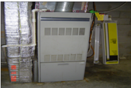
Oil fired furnace
