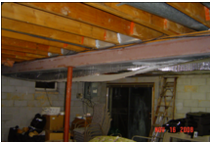
Insulation damage at duct
