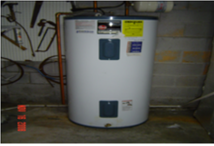
Existing water heater
